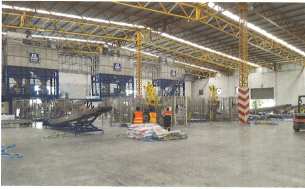
Figure 1. 6 x bagging lines for 25 and 50 kg bags installed in three bagging towers with a capacity of 6 x 40 tph.
