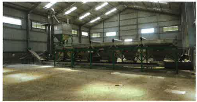
Figure 3. A five hopper Weighcont blender line and bagging line installed for ATA in Ethiopia, with a central capacity of 50 tph.
