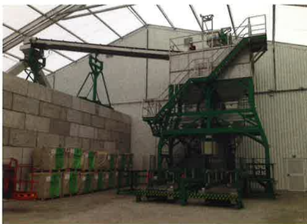
Figure 1. A high-speed twin big bag filling system installed in a Koch factory, France, with a capacity 140 tph for 500 to 1200 kg big bags.
