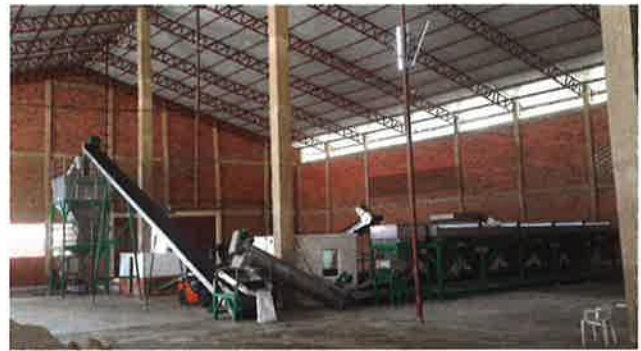
Figure 4. A five hopper Weighcont continuous blender line, which adds micronutrients, and a bagging line for 50 kg bags, installed in Rwanda.
