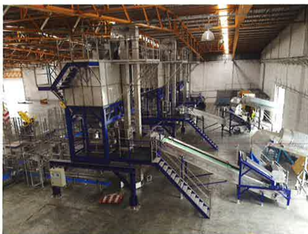
Figure 2. View of the Yara Thailand product intake machines with three elevators and three bagging hoppers with six bagging lines.
